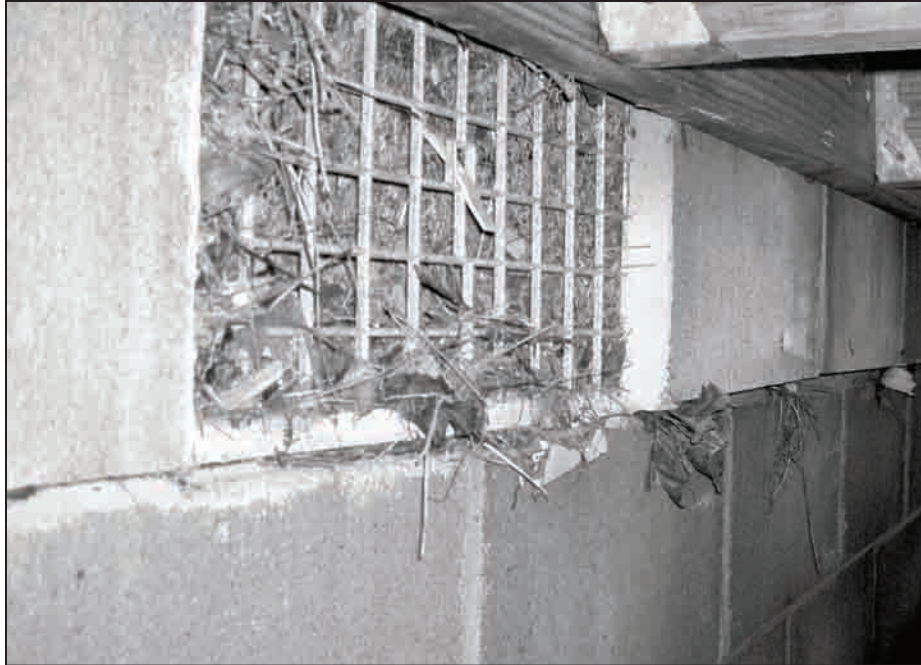
Figure 15. Typical air vent clogged by flood debris
