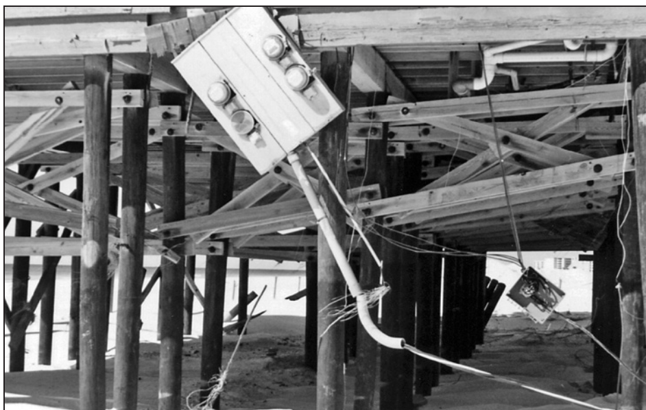
Figure 12-4. Electric service meters and feeders that were destroyed by floodwaters during Hurricane Opal (1995)
