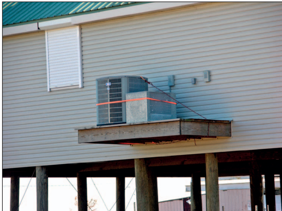
Figure 12-2. Proper elevation of an air-conditioning condenser in a floodprone area; additional anchorage is recommended
