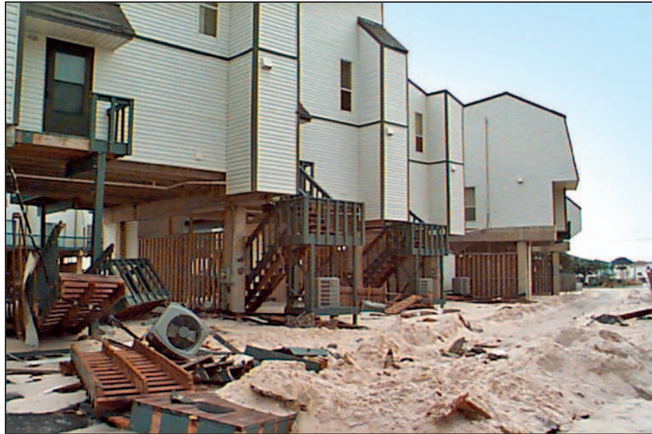
Figure 12-1. Condenser damaged as a result of insufficient elevation, Hurricane Georges (U.S. Gulf Coast, 1998)
