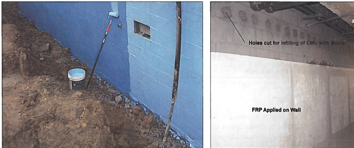
Figure 3-2. Application of a waterproof membrane on the exterior (positive side) of a wall (left) and fiber-reinforced polymer wrap applied to the interior (negative side) of a wall (right)
