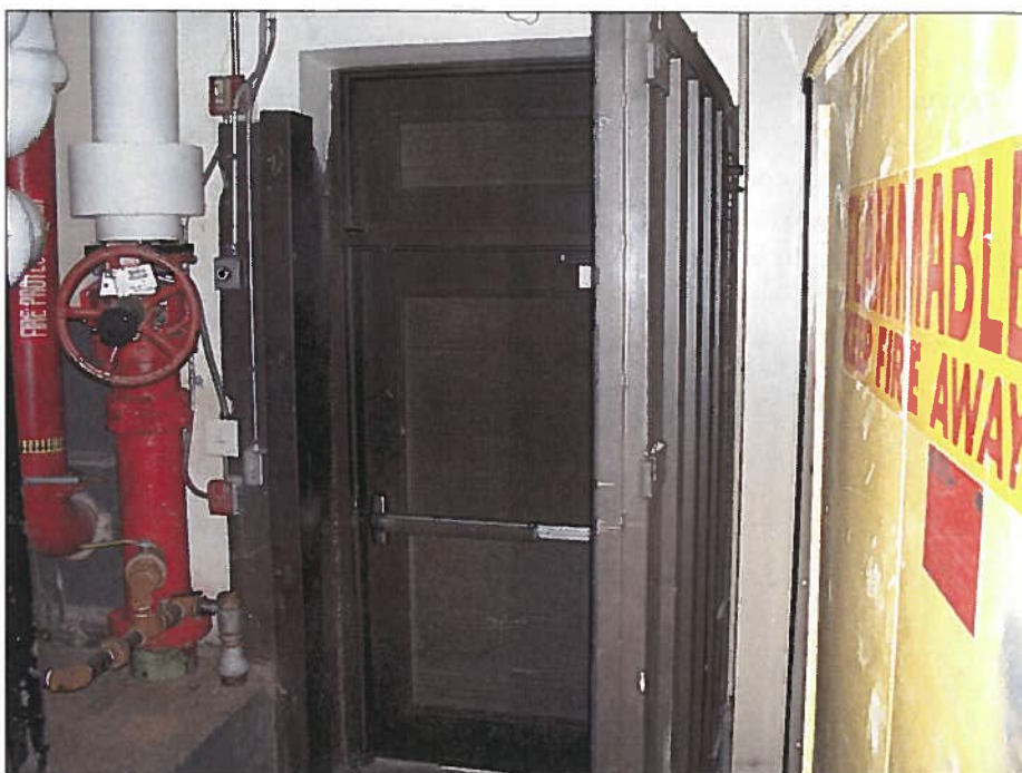
Figure 3-5. Watertight door used to protect mechanical rooms subject to flooding
