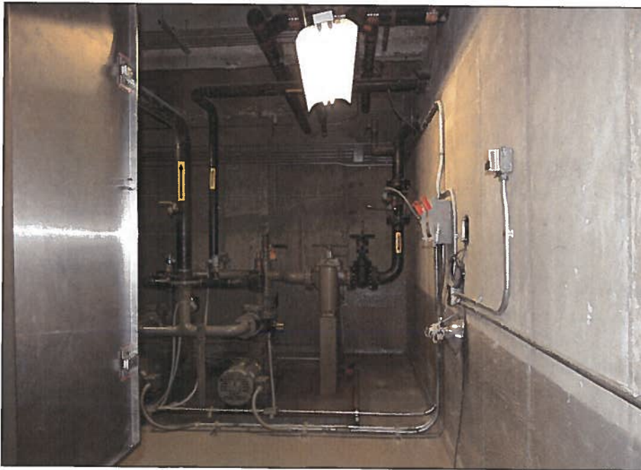
Figure 3-20. Dry floodproofed fuel pump room adjacent to generator fuel tank vault
